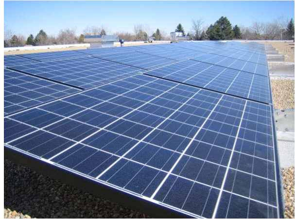
A 9.8 kilowatt photovoltaic system was installed on the roof of the new wing
